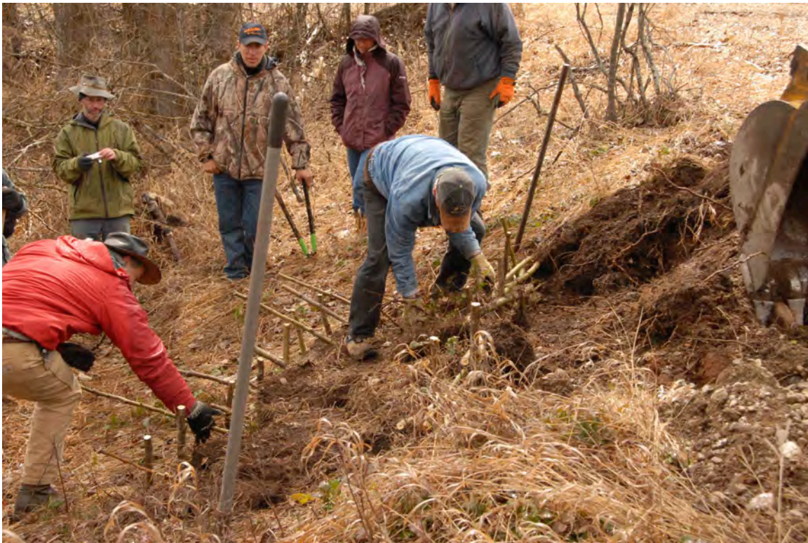
The brush layers are constructed with Cottonwood stakes, which will take root to stabilize the creek bank
